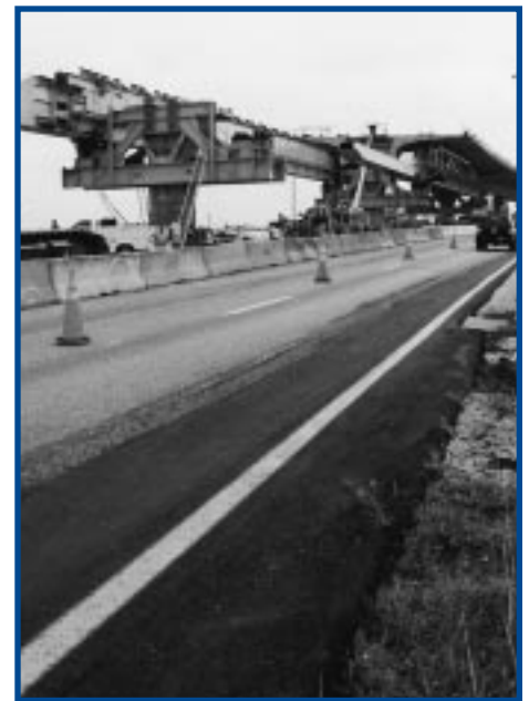
Traffic passes eastbound beneath several segments of the reversible bridge. The long beam in the foreground will be removed as more segments are put in place.
