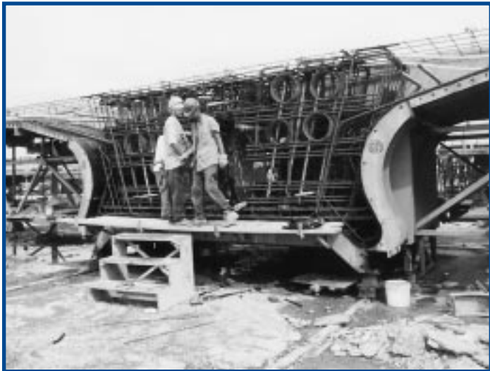
PCL employees standing in the hollow portion of a bridge segment form, prior to pouring the concrete, demonstrate the size of the core. The entire inside of the steel form is composed of various sizes and shapes of Gerdau Ameristeel reinforcing steel.
