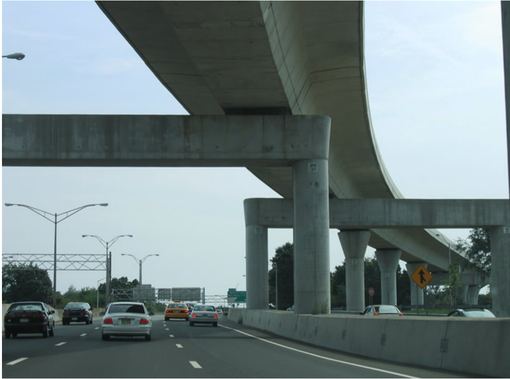
Photo of straddle bent supports under a New York highway. Notice that in the City rendering below how the sheer ugliness of straddle bent supports is minimized.
