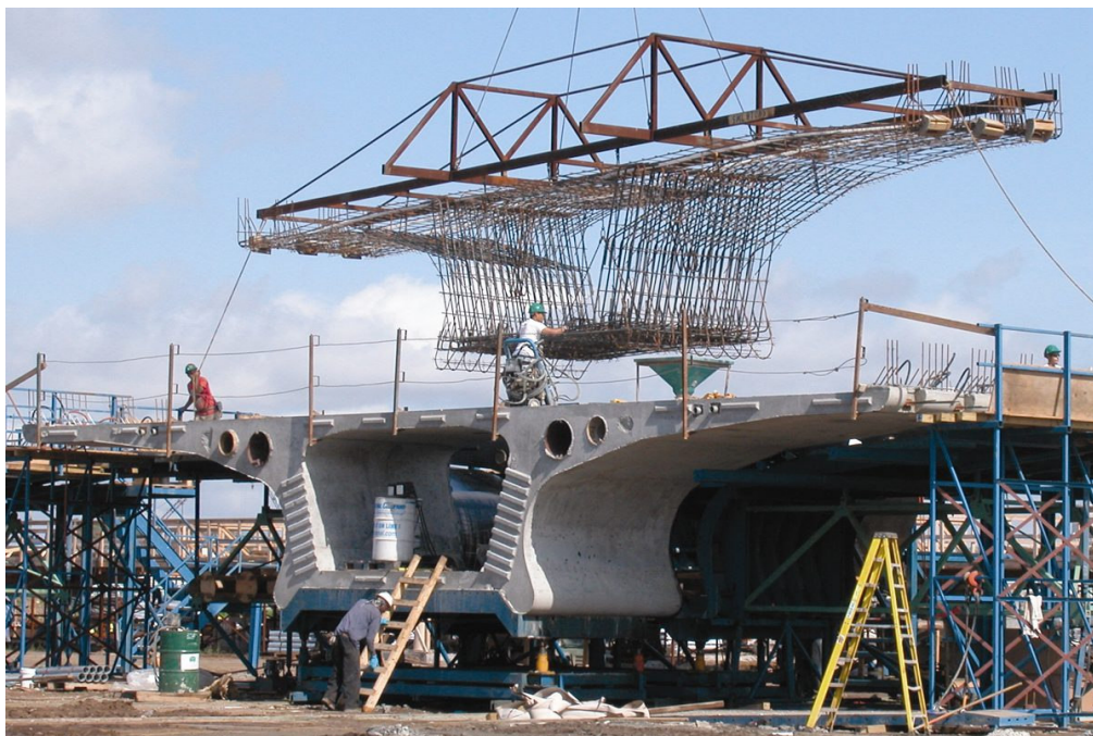
Figure C2. The segmental yard cast-matching technique was responsible for excellent on-site fit and large economies in construction.
